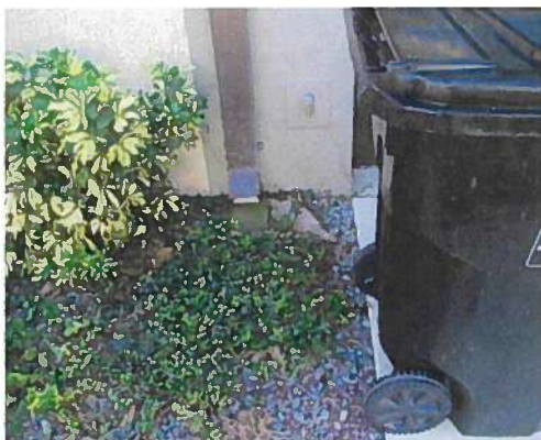
October 18, 2023, Disc PRE1, Photograph 158, JF, 6-unit building, downspout outlets at base of wall.
