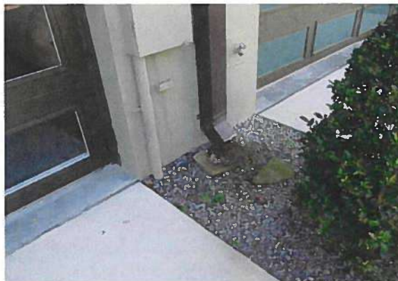
October 18, 2023, Disc PRE1, Photograph 159, JF, 6-unit building, downspout outlets at base of wall.
